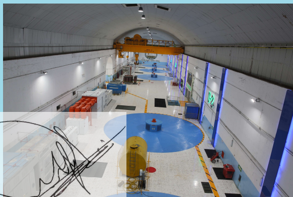
Hydroelectric Power Plants
